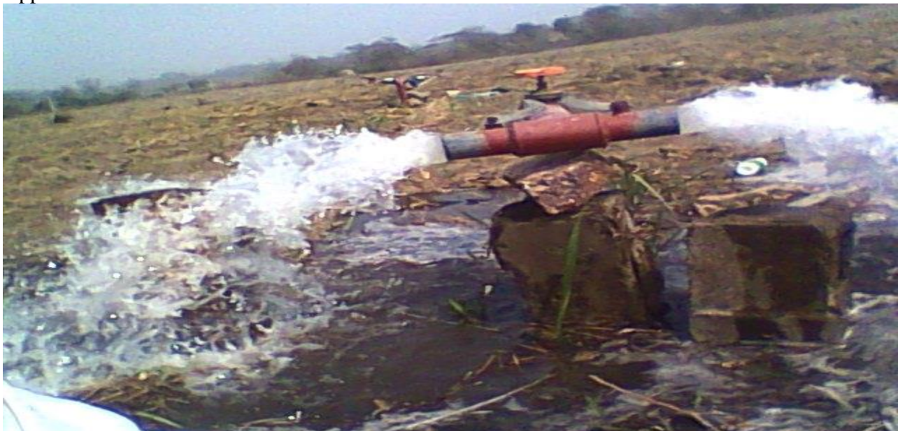
Central pump system at, Oke-Oyi, an irrigation scheme in the LNRBDA, before hoses were inserted
