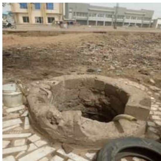
Plate 2: Well located at filthy (Defecated)
