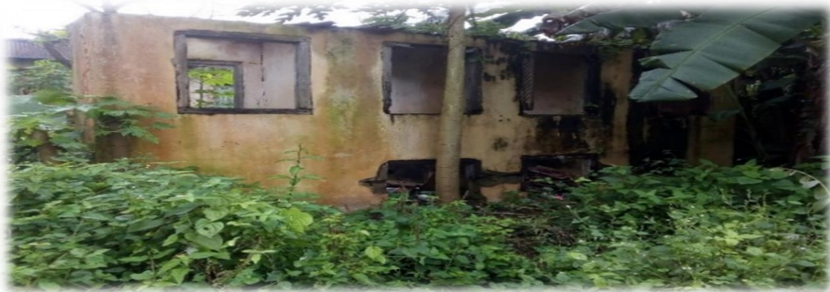
Plate 2.2: A dilapidated bucket latrine
