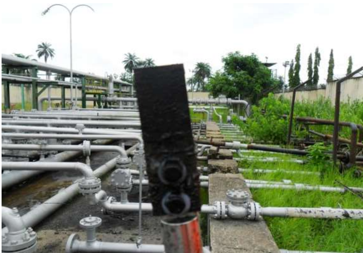
Fig 3: Biofilms on coupons after 127 days in oil Pipelines
