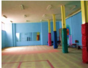
Figure 22. High school gymnasium in poor quality (Abnieh Tarrahan Alborz, 2008)
