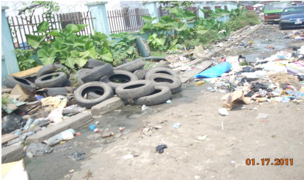
Plate 4.3: A Drain Blocked with Waste and on the Street at Coronation Layout.
