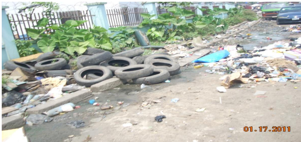
Plate 4.3: A Drain Blocked with Waste and on the Street at Coronation Layout.
