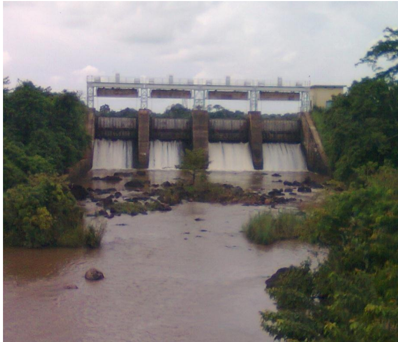
Figure 1: Downstream side of the spillway with fractured floor
