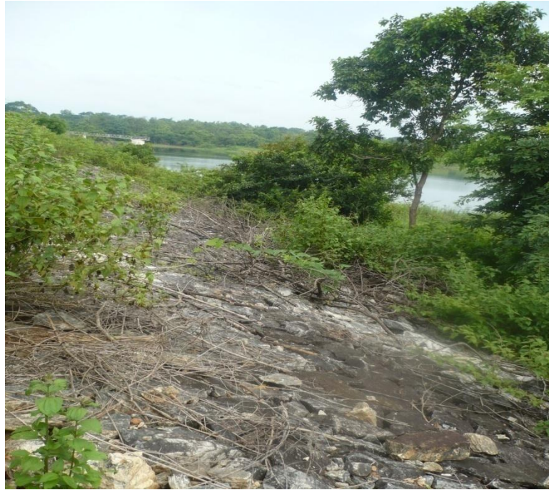
Figure 5: Dislocated stone riprap with tree vegetation at upstream side
