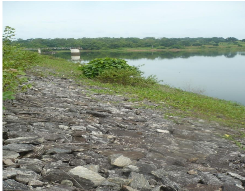
Figure 6: Disjointed stone riprap at upstream side
