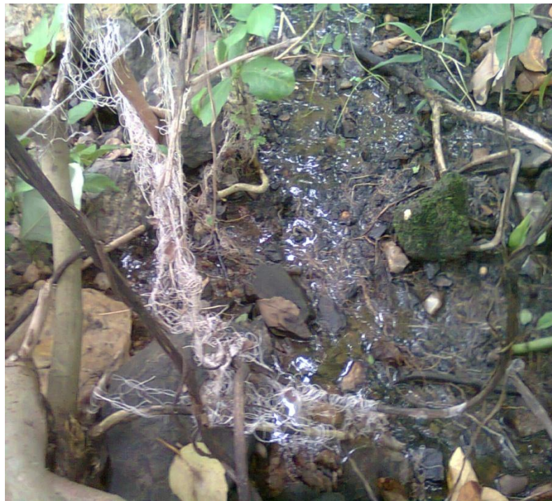
Figure 2: Seepage water flowing out at downstream toe
