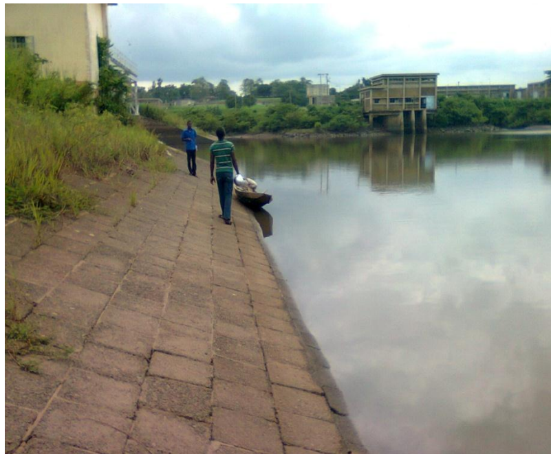
Figure 4: Disjointed concrete slabs at upstream face
