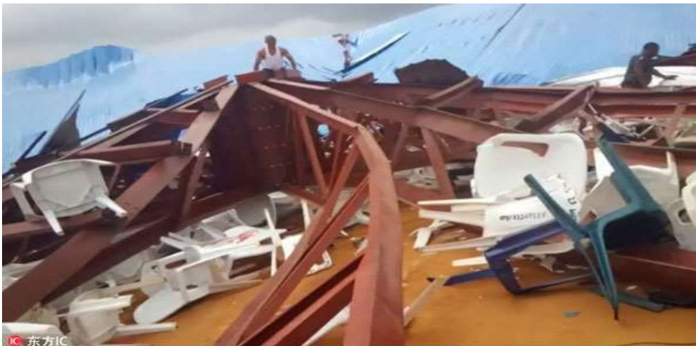
Fig 1 photo of collapse Reigners Bible Church Building
