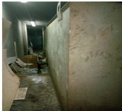
Plate 7: leakages in the basement
