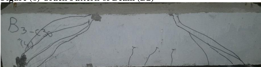
Figure (7) Crack Pattern of Beam (B3)
