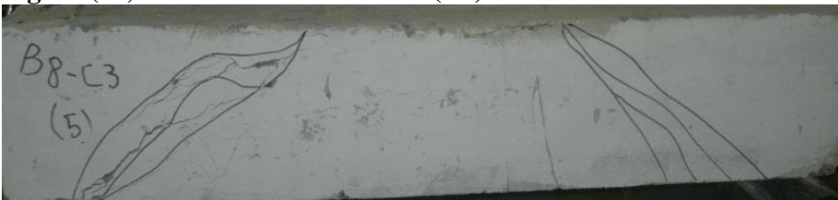
Figure (12) Crack Pattern of Beam (B8)
