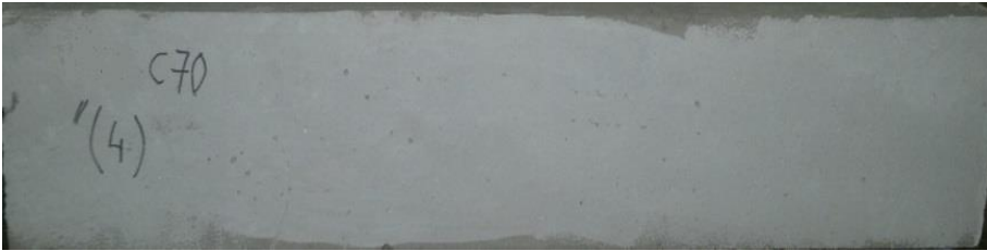
Figure (9) Crack Pattern of Beam (B5)
