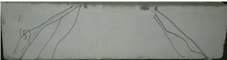
Figure (5) Crack Pattern of Beam (B1)
