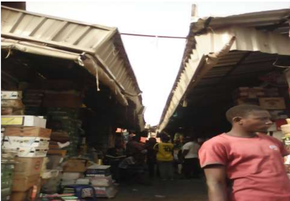
Plate IV: Lock-up Shop Buildings in the Market in FCT with Inadequate Spaces between them (Source: Researchers' Field Work, 2020).
